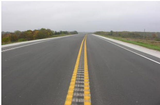
Centerline Rumble Strips
