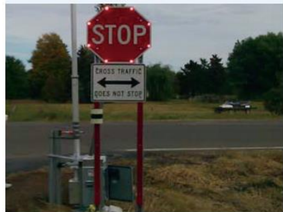
Figure 3-9. Light-emitting Diode Stop Sign
