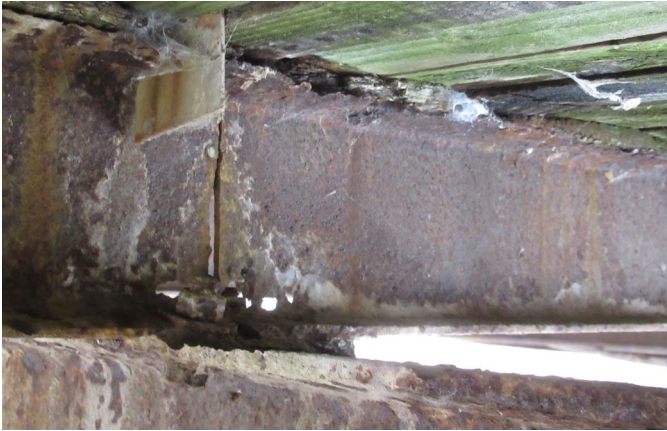
Stringer & Floorbeam Corrosion
